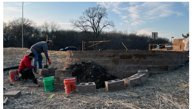
Liam Dempsey and Trenton Franz work on building the Hole 10 gold tee area featuring a multi-tiered retaining wall. Native shrubs and arborvitae trees were added to the tee area in the spring.
